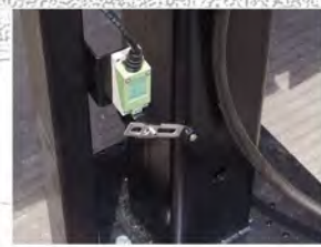
Lower limit switch
